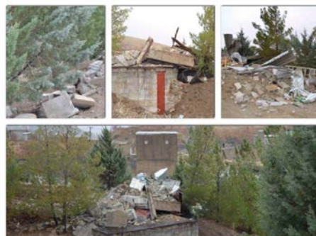
Images of the destruction at the Bahá’í cemetery in Sanandaj, Iran, which occurred on 12 December 2013
