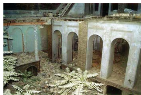
Interior of the house of Bahá'u'lláh's father, Mirza Abbas Nuri, an architectural landmark in Tehran, during its demolition in June 2004.
