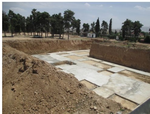
Iranian Revolutionary Guards building a sports and cultural complex over a Bahá'í cemetery. This photo shows concrete being poured into the site where the graves of Bahá'ís were excavated in order to lay the building foundation.
