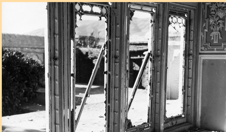
Interior of the historic 19th century home of the Báb after its 1979 destruction (Credit: Bahá'í International Community)
